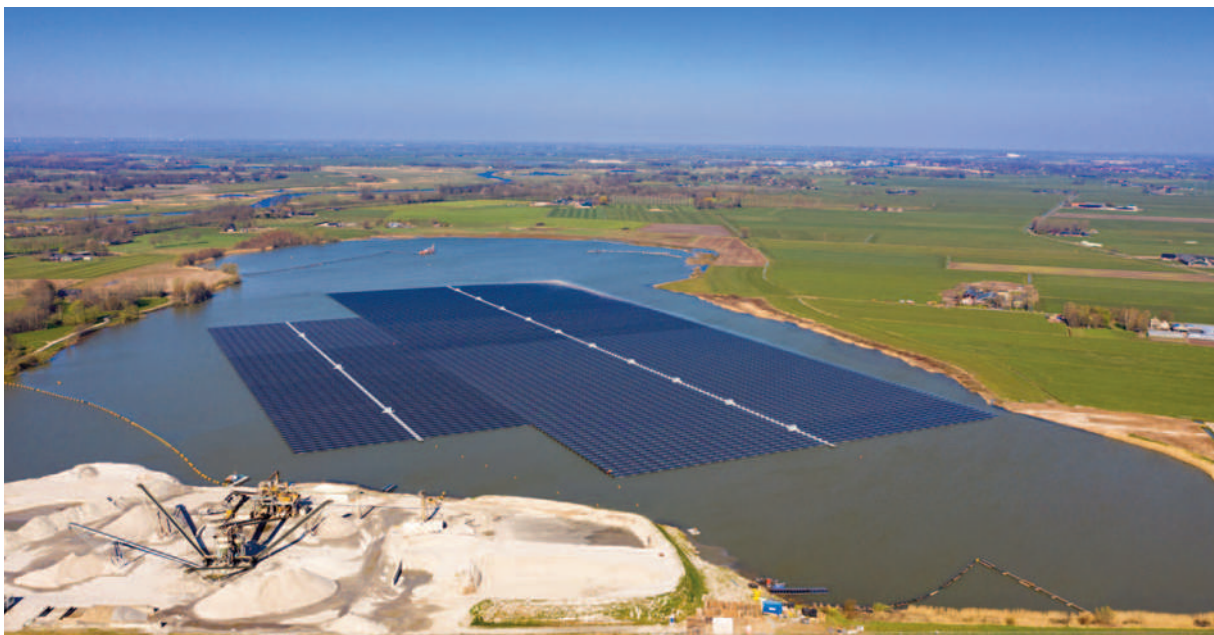
27.4 MW, Bornhofspas, the Netherlands.
