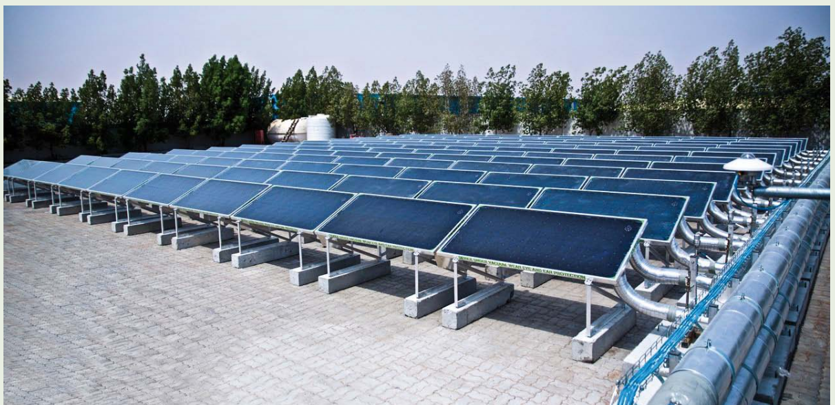
High vacuum flat plat collectors at a rubber factory in Ras Al Kaimah, United Arab Emirates
