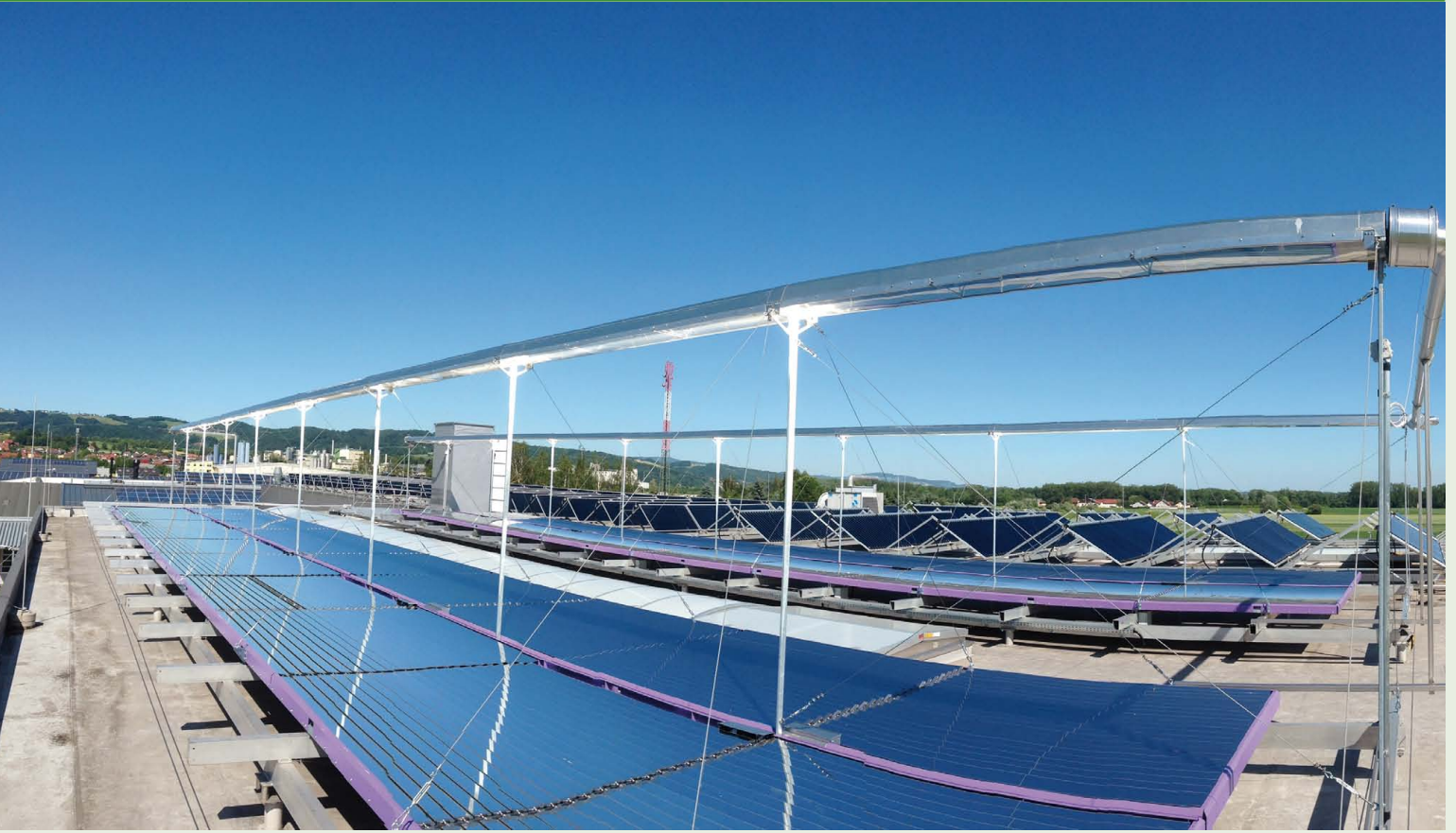
Linear concentrating Fresnel collector system in Austria.
