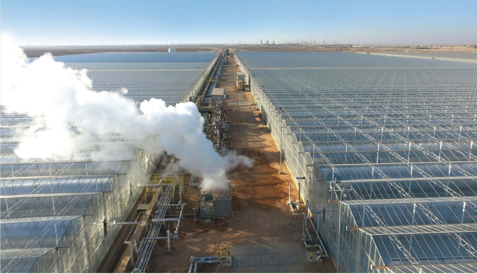
The world's largest solar process heat plant Miraah in Oman was significantly enlarged in 2019 and now has an installed capacity of 300 MW th .
