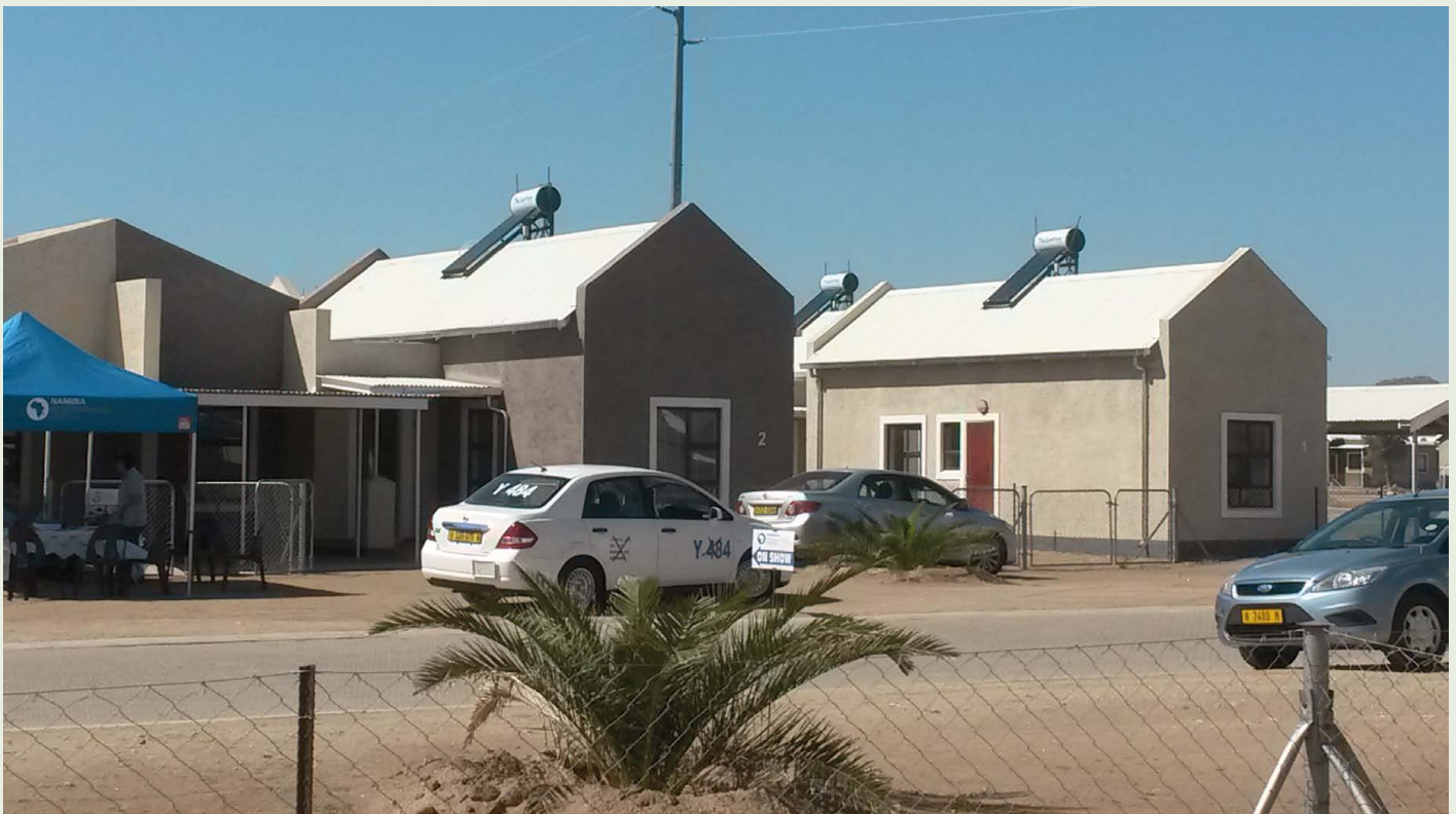
10,000 apartments in Osona Village, Namibia are being equipped with thermosiphon systems.
