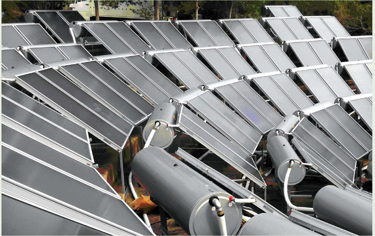
Greek thermosiphon systems
