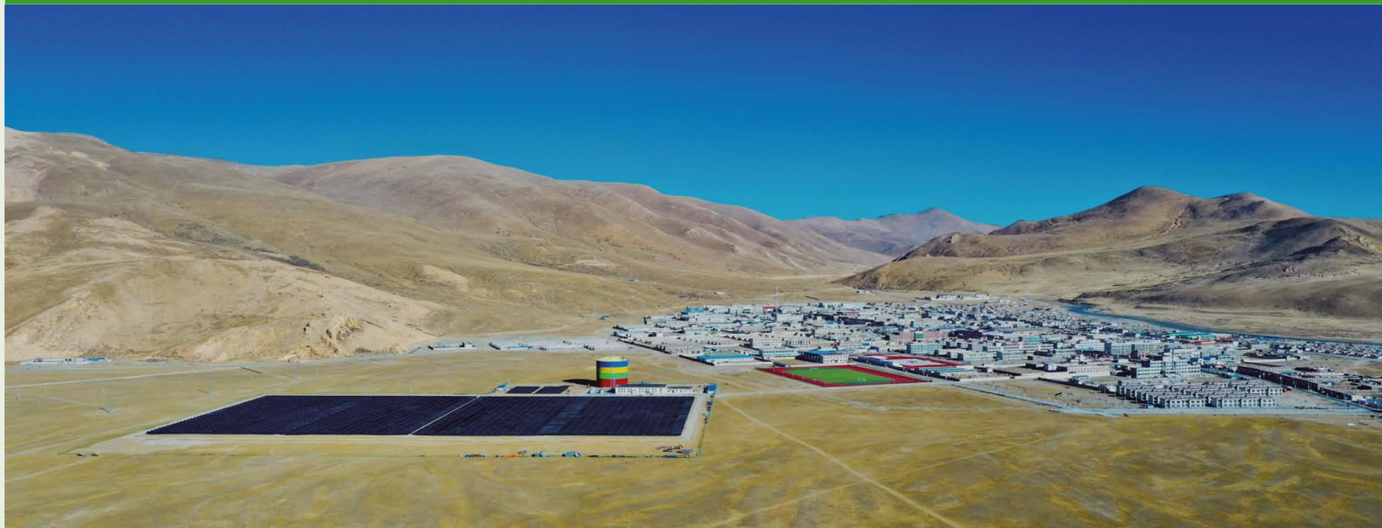
The Zhongba solar district heating system in Tibet, China with 35,000 m 2 collector area (24 MW th ).
