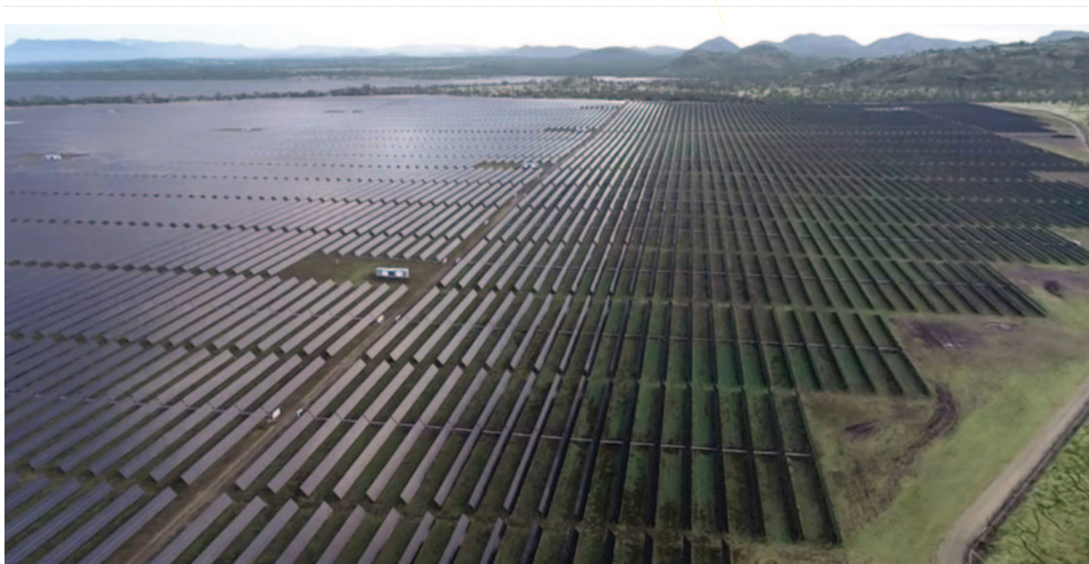
Daydream Solar Farm , 180 MW, Queensland.
